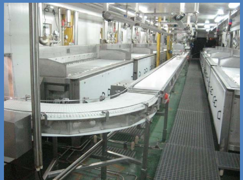
Picture of the units installed on board.
